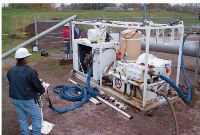
Figure 3. Pumps, such as the one shown here, are used to fill a line section with water in advance of hydrotesting.
